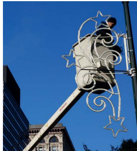
NOVEMBER USP installs 80 holiday lights to brighten the district during the holiday season.
